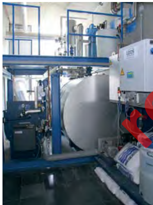
Figure 126: Steam generator of the company LOOS at the FRAUNHOFER IFAM (COPYRIGHT) in Bremen
