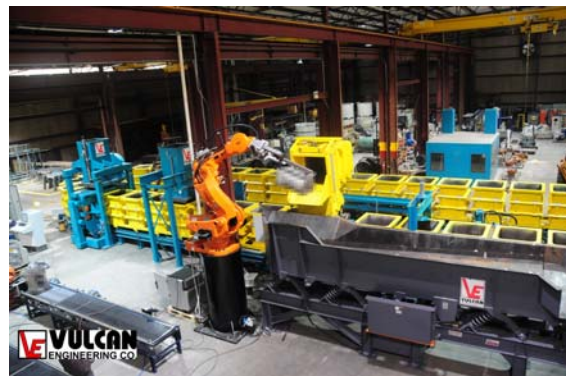
35 FPH Aluminum Line to Produce Truck Parts w/ 1 Hour Cooling Note the Casting Extraction Robot
